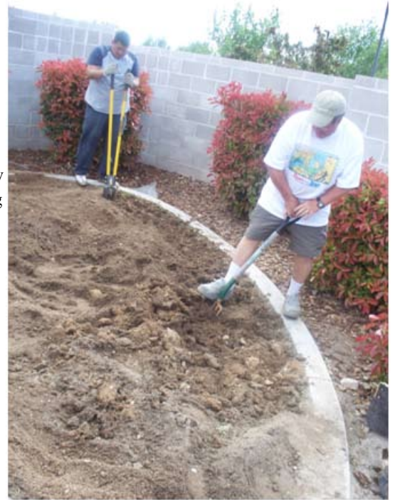
Jerry Etheridge and John Reams get the ground ready to plant a wildflower garden at the Family Enrichment Center playground
